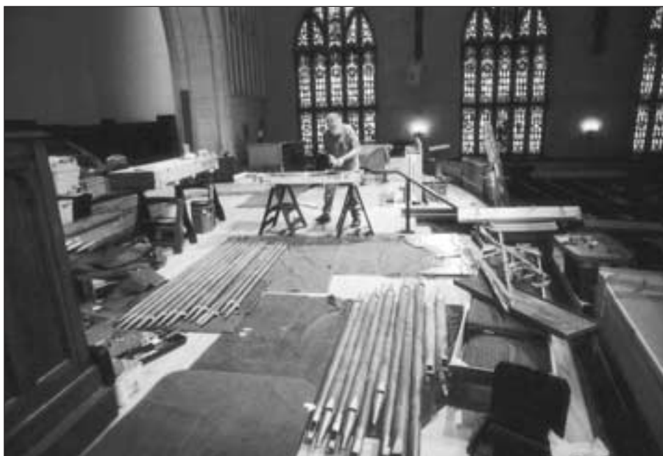
In January, the Thompson-Allen Company began dismantling the organ so that it can be shipped to New Haven, Conn., for restoration. The removal will continue in March. The organ is due back in time for Vespers at the end of the year.
