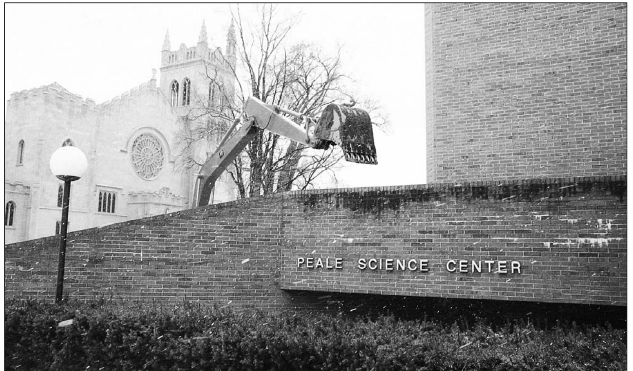
Munch. As work begins on the new science center in March, bites are taken out of the berm on Peale Science Center's east side for a new lower entrance.
