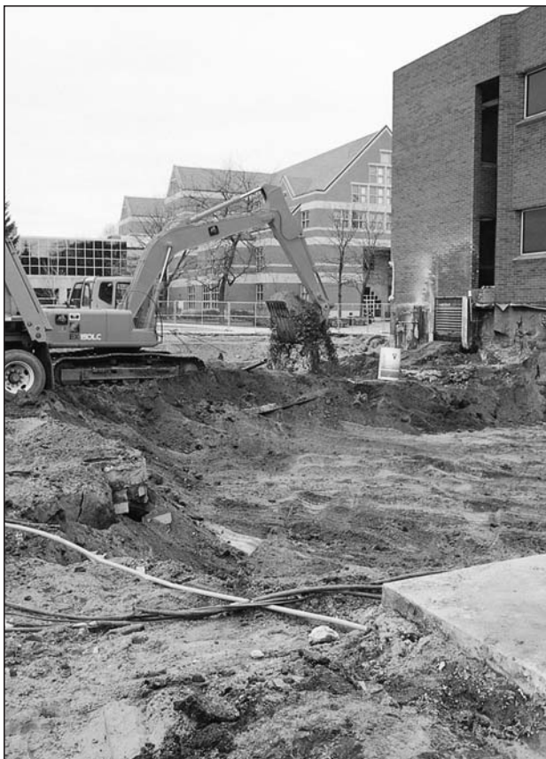
Digging out the lower level of the new science center. Images from a live Web cam (refreshed every minute or so) showing work at the site can be viewed on-line at: www.hope.edu/academic/natsci/building .
