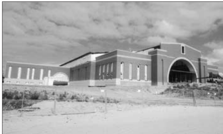
Work continues on the DeVos Fieldhouse, which will open for the 2005-06 basketball season.
