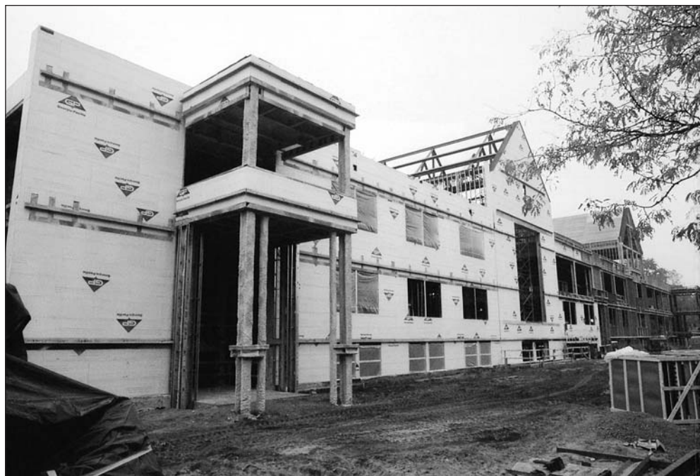
The science center continues to progress rapidly, with roof plating and walls replacing open girders.
