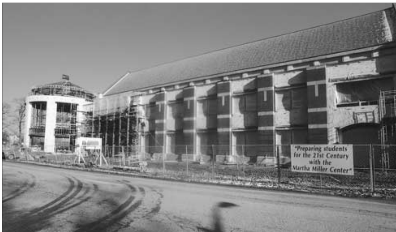
Burgeoning brickwork adds a hint of finish to the Martha Miller Center for Global Communication, which will house the departments of communication and modern and classical languages, and the offices of international education and multicultural life.
