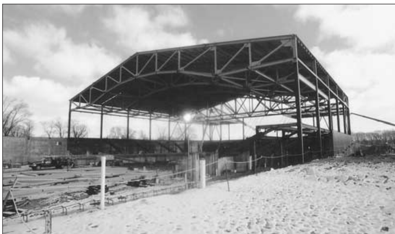
A spectator facility designed with the entire community in mind, the DeVos Fieldhouse takes shape as the steelwork sprouts from the poured concrete walls. The building will be home court for men's and women's basketball, and will house the department of kinesiology and the athletic training program.
